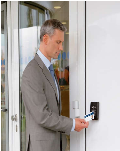
Physical access control
